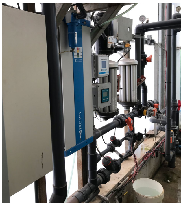
Figure 16. Reverse osmosis filtration system.
