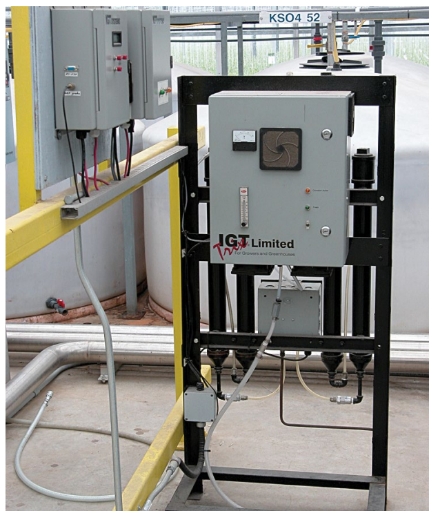
Figure 21. Ozone disinfection system.
