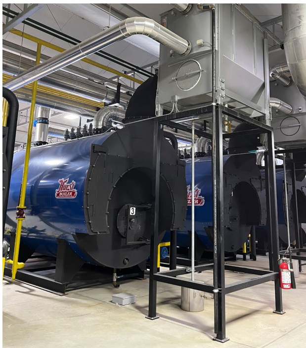
Figure 11. Natural gas boiler (bottom portion) with flue gas scrubber (top portion) to provide heat and CO 2 for greenhouse vegetable production.
