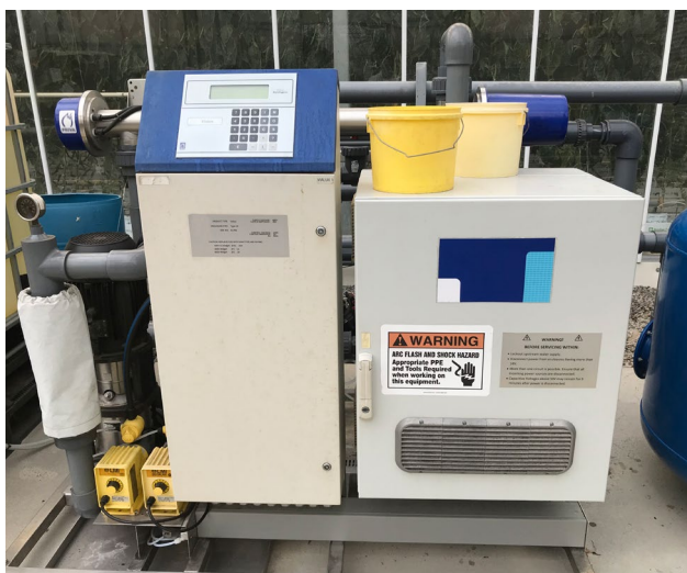
Figure 20. UV disinfection system.
