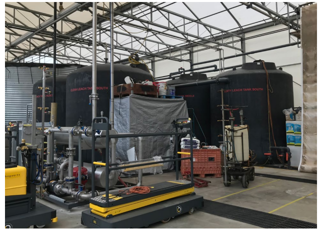
Figure 19. Heat (Pasteurization) disinfection system (left) and clean and dirty water tanks (right).
