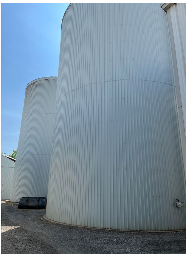
Figure 36. Hot water storage tanks.
